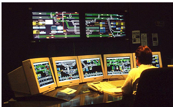
The “Advanced Train Running Information Control System” (ATRICS) developed by Rail Infrastructure Corporation is now used for the control of the new Airport line and the Olympic loop, and Stage 1 of its possible wider introduction, controlling a number of other areas from Sydenham, is underway.
